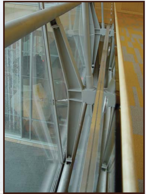
Close-up view of the typical tension rod connection for the glass walls.
